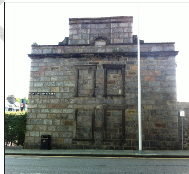
Example of blocked up windows in Ferryhill
